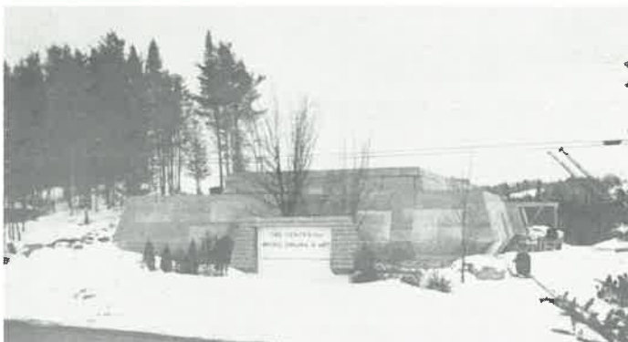
Under construction, the new Arts Library for the Lake Placid Center for Music, Drama and Art.
